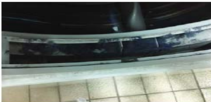
Filter chamber also getting blocked by lint
